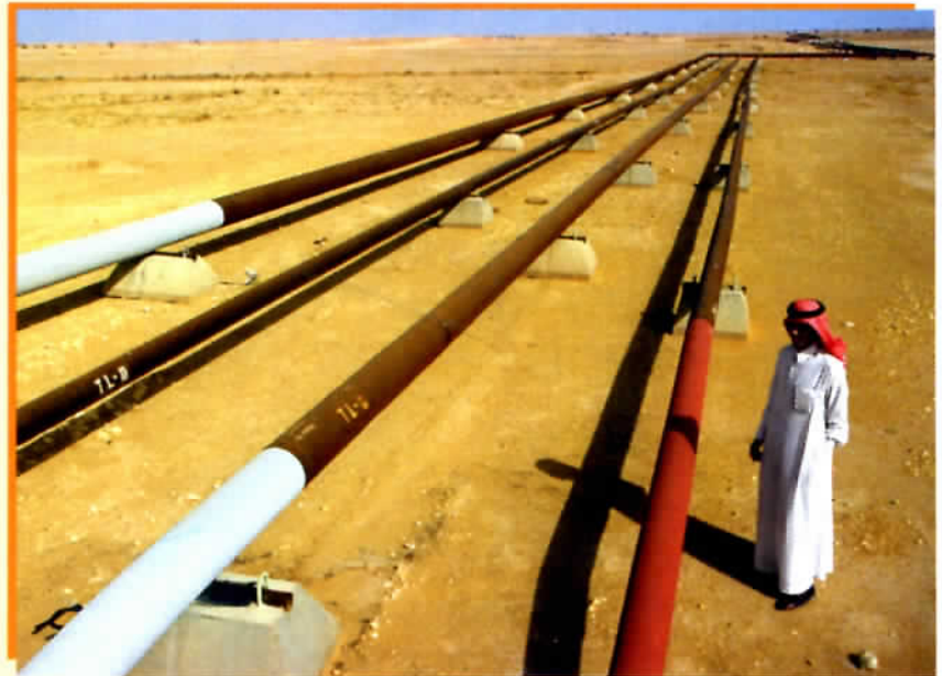
Pipelines carry oil many miles across the Saudi Arabian desert to ports on the Persian Gulf and the Red Sea.
